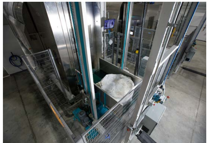
A LAVATEC press removes excess moisture, and the linen “cake” goes to the next available dryer.
